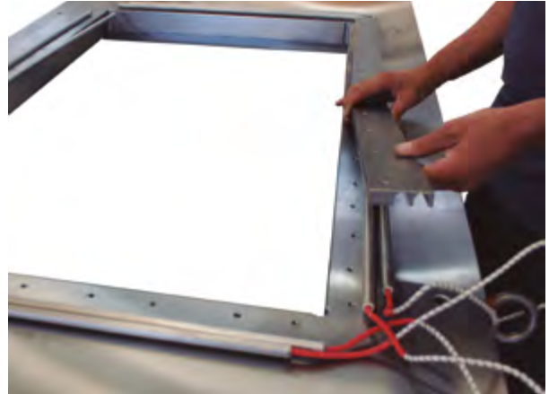
Figure 3.63. L-shaped perimeter heating elements.
