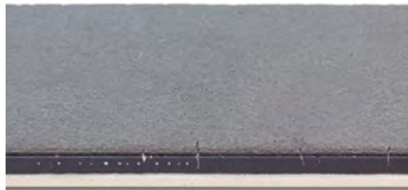
Figure 7.25. Comb or bevel cracks.
