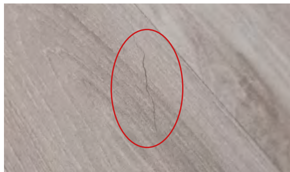
Figure 7.22. Central crack due to uneven cavity loading.
